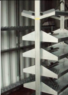
Detail of racks
