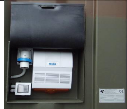
Detail of exterior with: electrical junction, alarm switch – internal light switch and siren with flashing light
