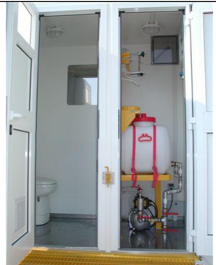
View of the front technical compartments
