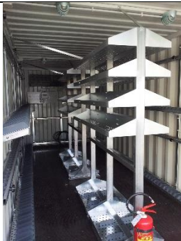
Detail of racks
