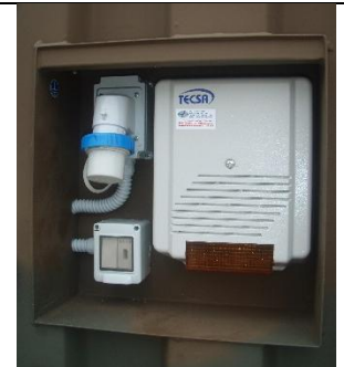
Detail of exterior with: electrical junction, alarm switch – internal light switch and siren with flashing light
