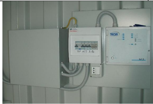
Detail of electrical panel (interior) and alarm box
